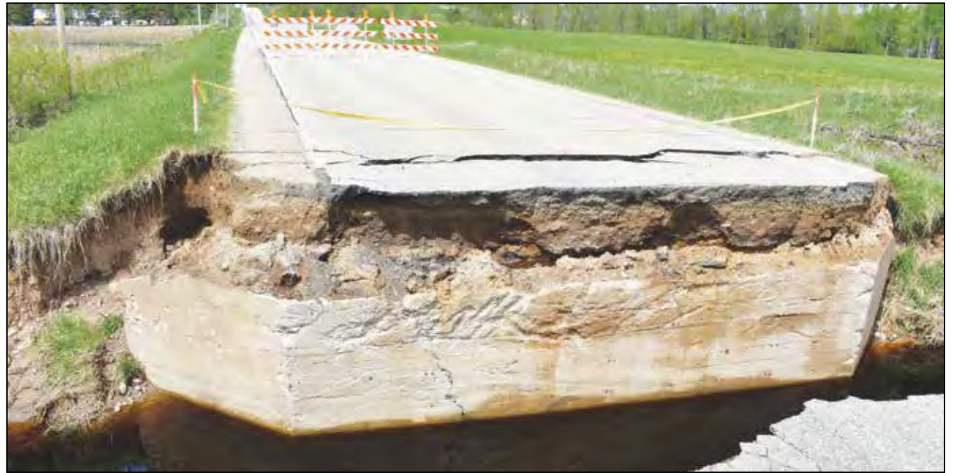
A portion of County Road B north of Yatso Road is expected to remain closed for several weeks after flood waters washed out a culvert during severe thunderstorms May 12.
