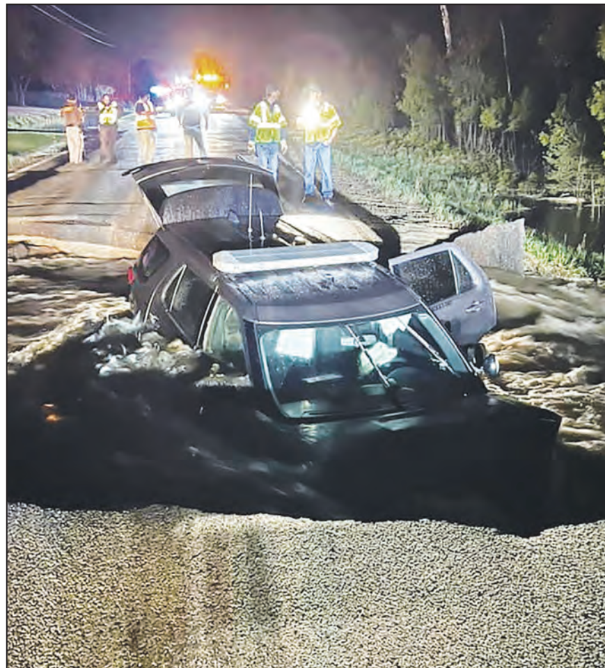
An Oconto County Sheriff's Department squad car was wrecked May 12 when the pavement on County Road A gave way as he drove over a culvert that had been compromised by rushing flood waters. He and his K-9 partners escaped without injury, but the road remained closed for weeks.
