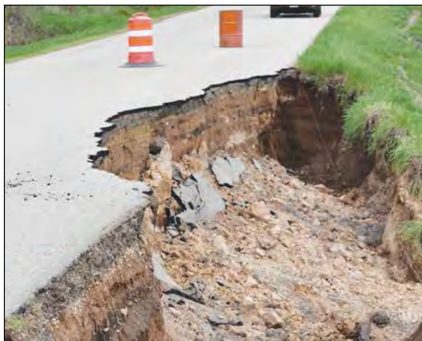
Flooding from a severe thunderstorm May 12 caused several roads to wash away, including a portion of Brock Road in the Town of Maple Valley.
