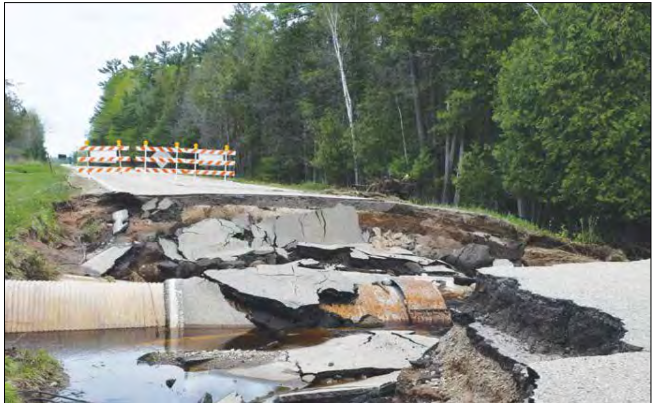
A portion of County Road A in the Town of Maple Valley remained closed May 15 after a culvert gave way under the pavement three nights earlier.
