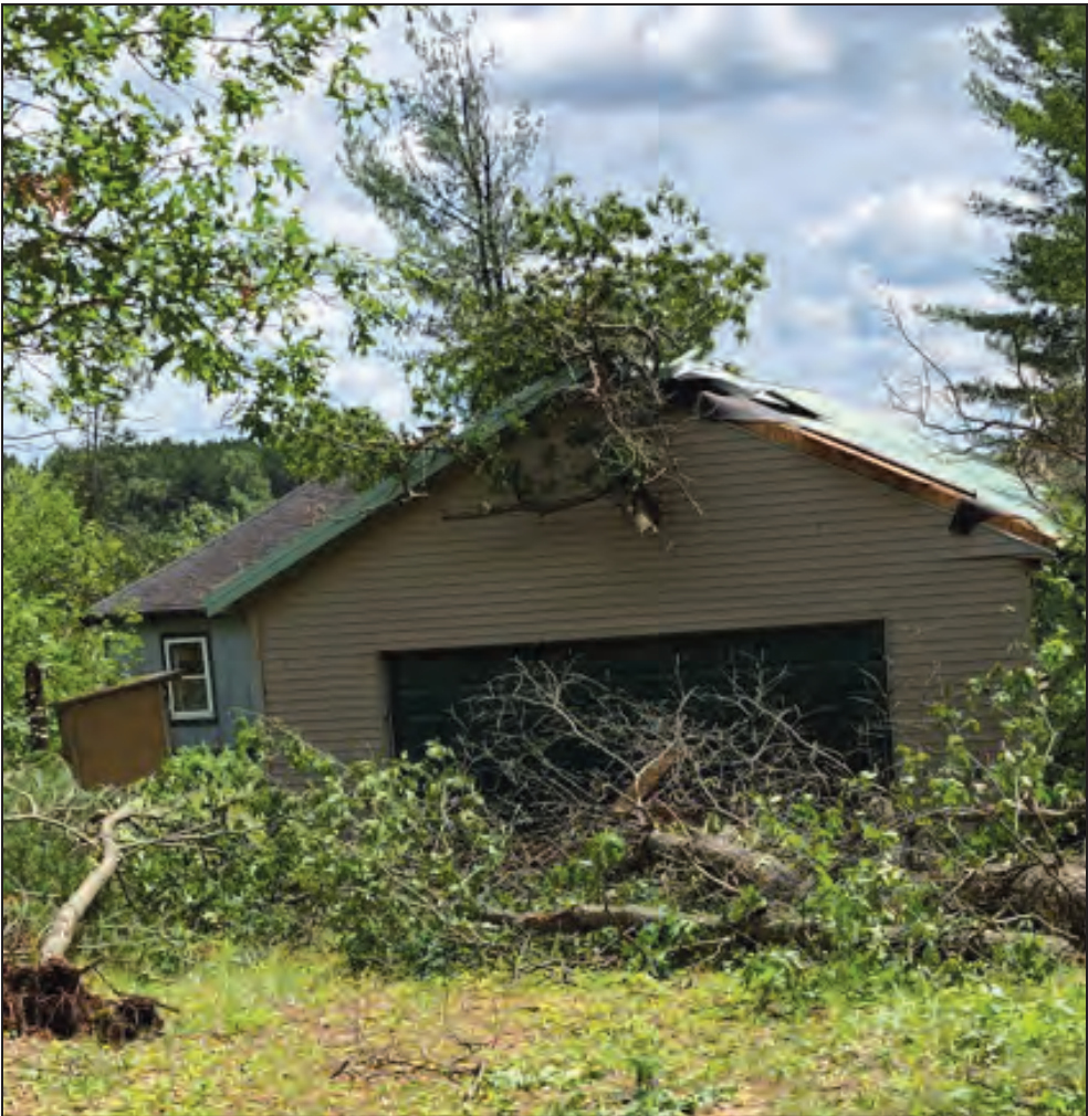
Trees were snapped in half and power outages were common in the area when severe storms struck the night of June 24-25.
