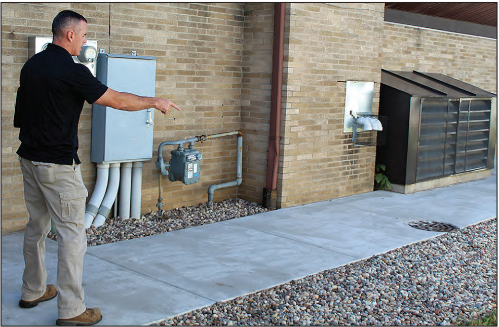
Grant Bystol, Shawano County highway commissioner and a member of the county's ad hoc building committee, points to an area his staff repaired on the north side of the Shawano County Library. The committee will eventually recommend a course of action regarding the library, courthouse, jail and sheriff's department — to continue the existing maintenance plan, renovate or build new.
